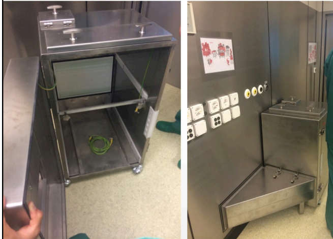
Separating heater-cooler unit from operating room air
