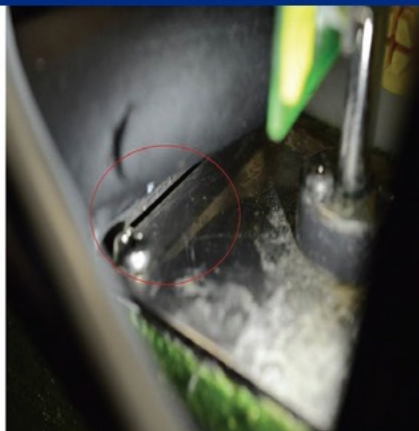
Gap in water tank sealing plates
